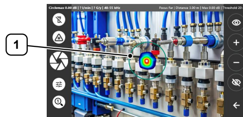
Figure 17: Leakage optimally detected (example)
